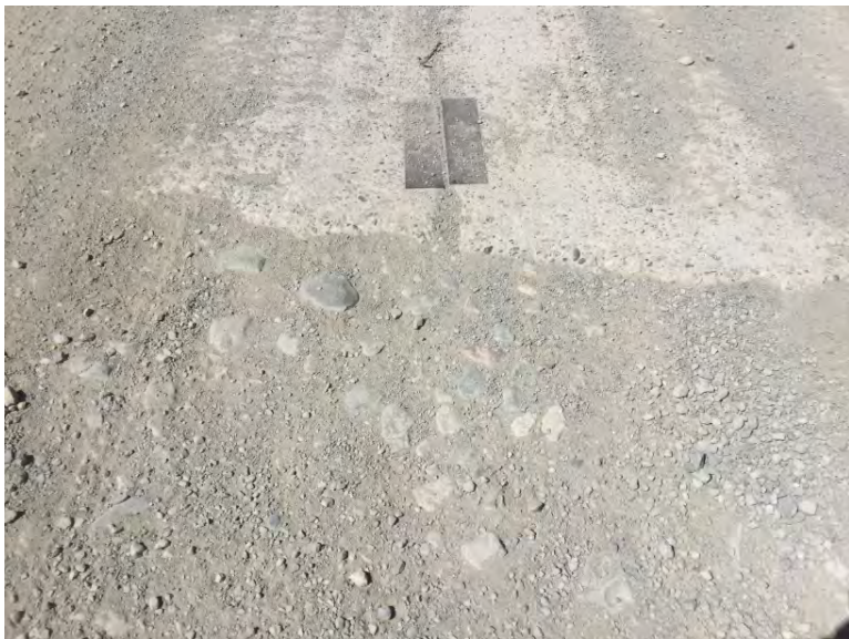
Minor damage to slab ends at right bank
